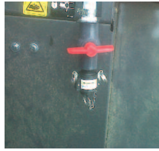
Filling and drain point
